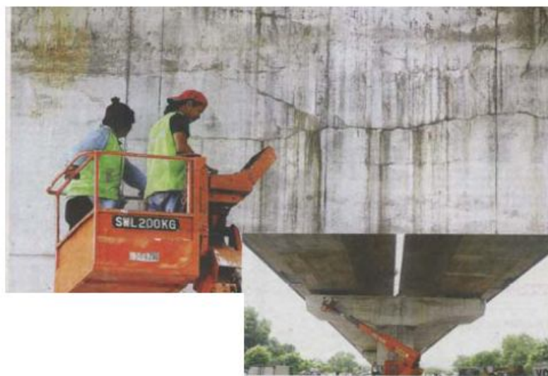
Fig. 6.4: Crack Pattern in Bridge [4] .
