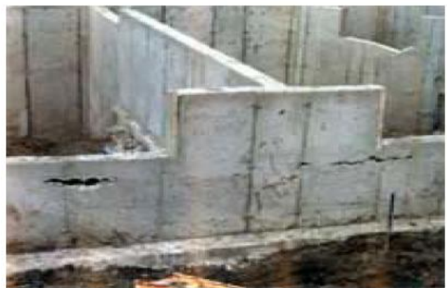
Cold Joints ( www.enhance-solutions.com )
