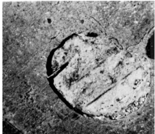
(b) Large Spall
