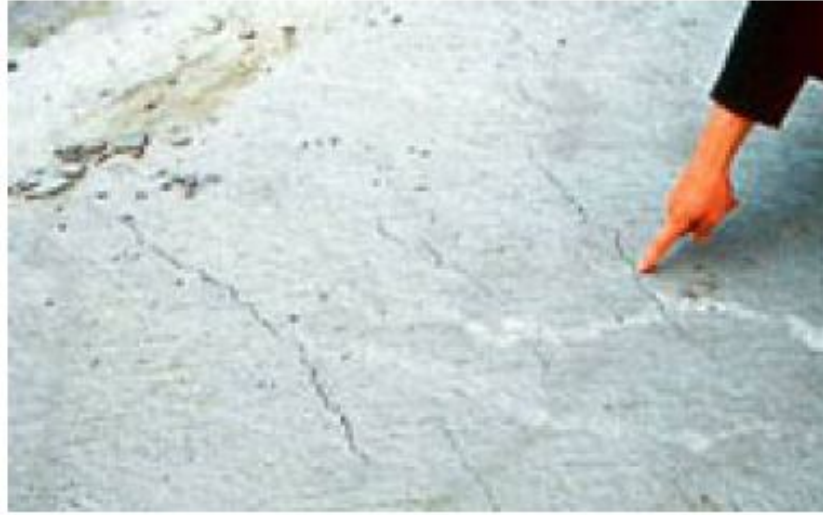
Fig. 3.2: Plastic shrinkage cracks. ( www.cement.org/tech/faq_cracking.asp )
