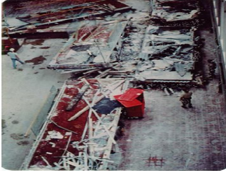
Fig. 6.1: photo of walkway section taken from second floor opening. Walkway section still remained as a piece-form [4] .
