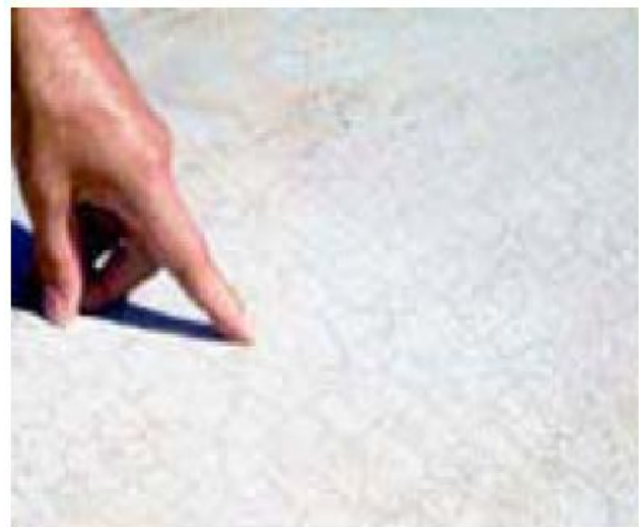
Fig.3.4: Craze cracks. (www.praire.com)
