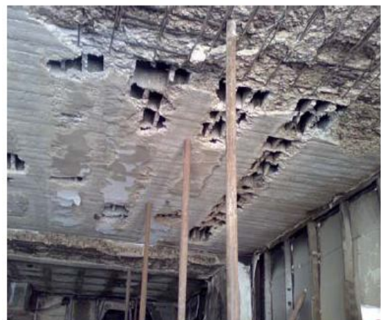
Fig.3.7: Typical fire damages (IUG library building- march )
